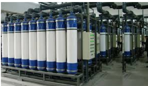
Ultra Filtration System
