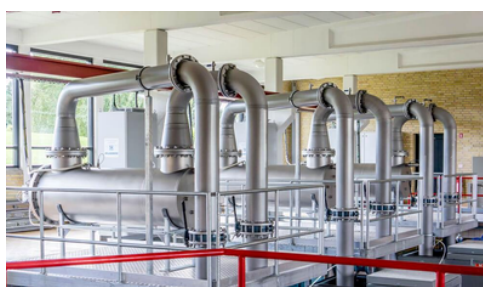
UV disinfection System
