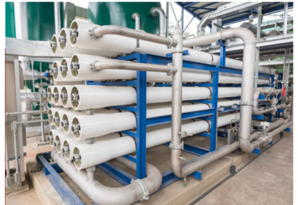
Brackish Water Reverse osmosis system
