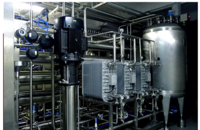
Electro Deionisation/demineralisation system
