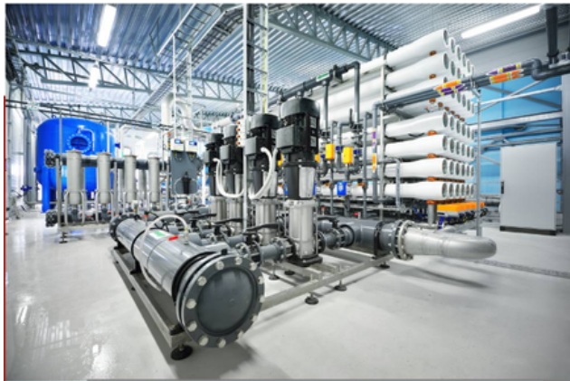
Sea Water Reverse Osmosis System
