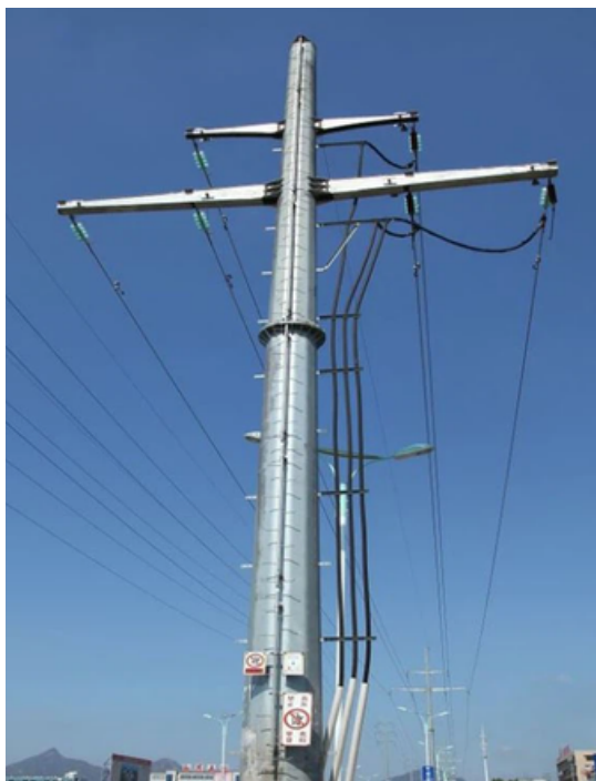
Low Voltage /High Voltage Transmission Pole
