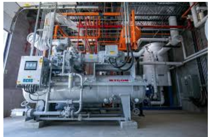
Ammonia Refrigeration System
