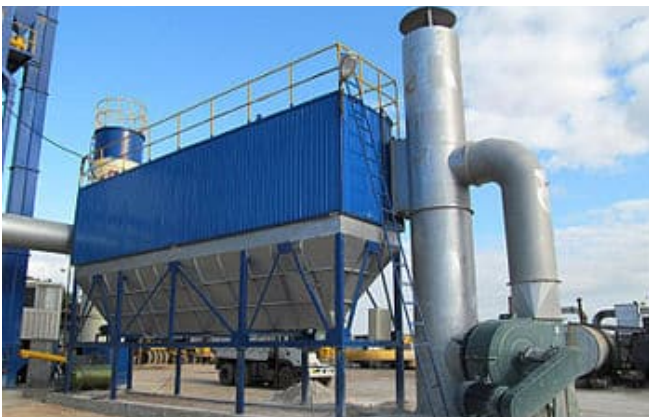
Dry Dedusting System
