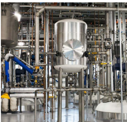
Chemical Filtration Equipment
