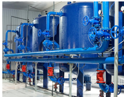
Zero Liquid Discharge system
