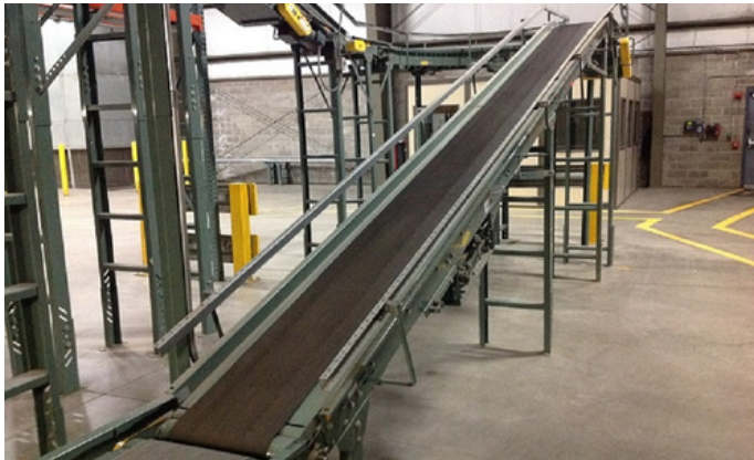
Belt Conveyor system
