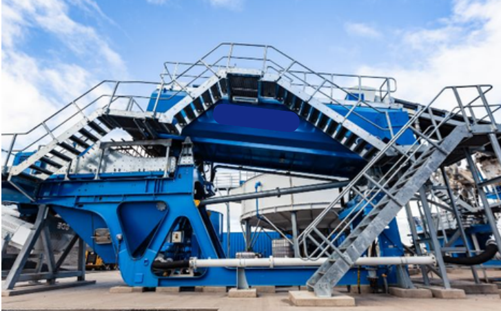
Scrubbing & Classification system
