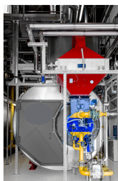
Air Preheat System
