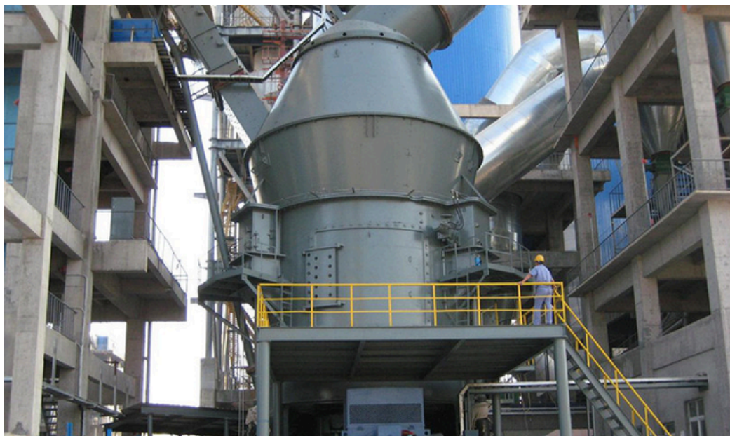
Cement Clinker Milling Plant
