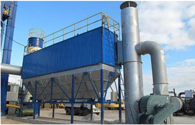
Dry Dedusting System
